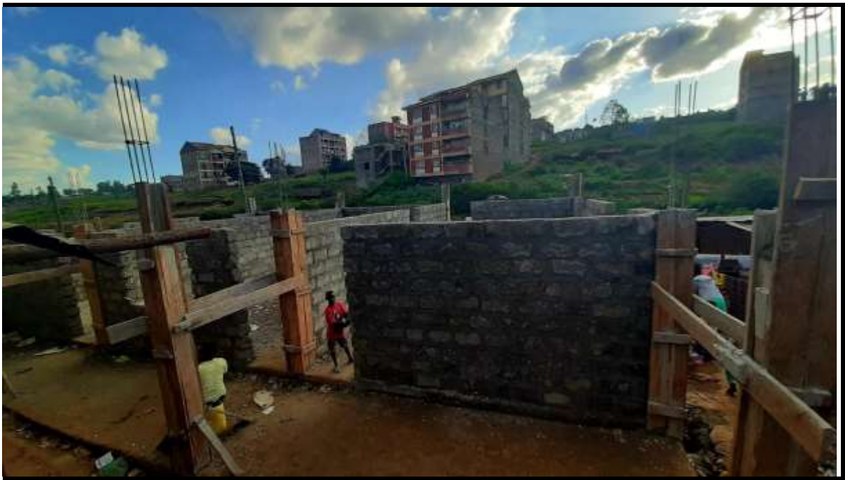
3 classrooms are put in place in the Ground floor (End of October 2020)
