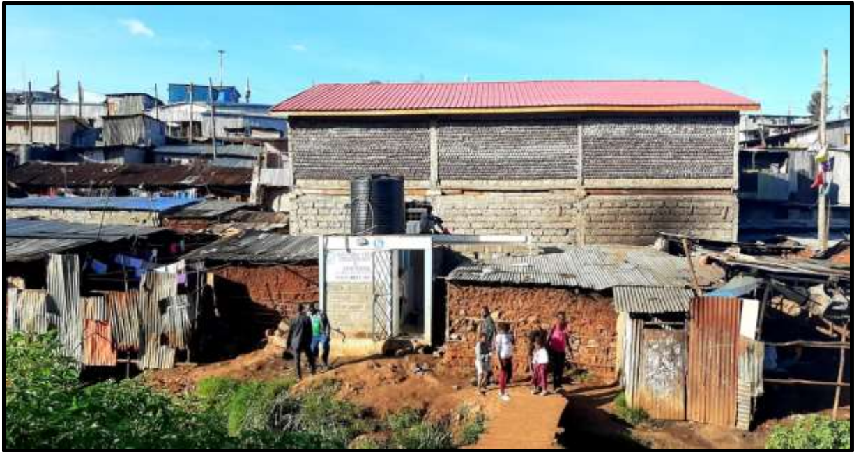
Building of a front wall made with recycled plastic bottles (Mid March 2021)
